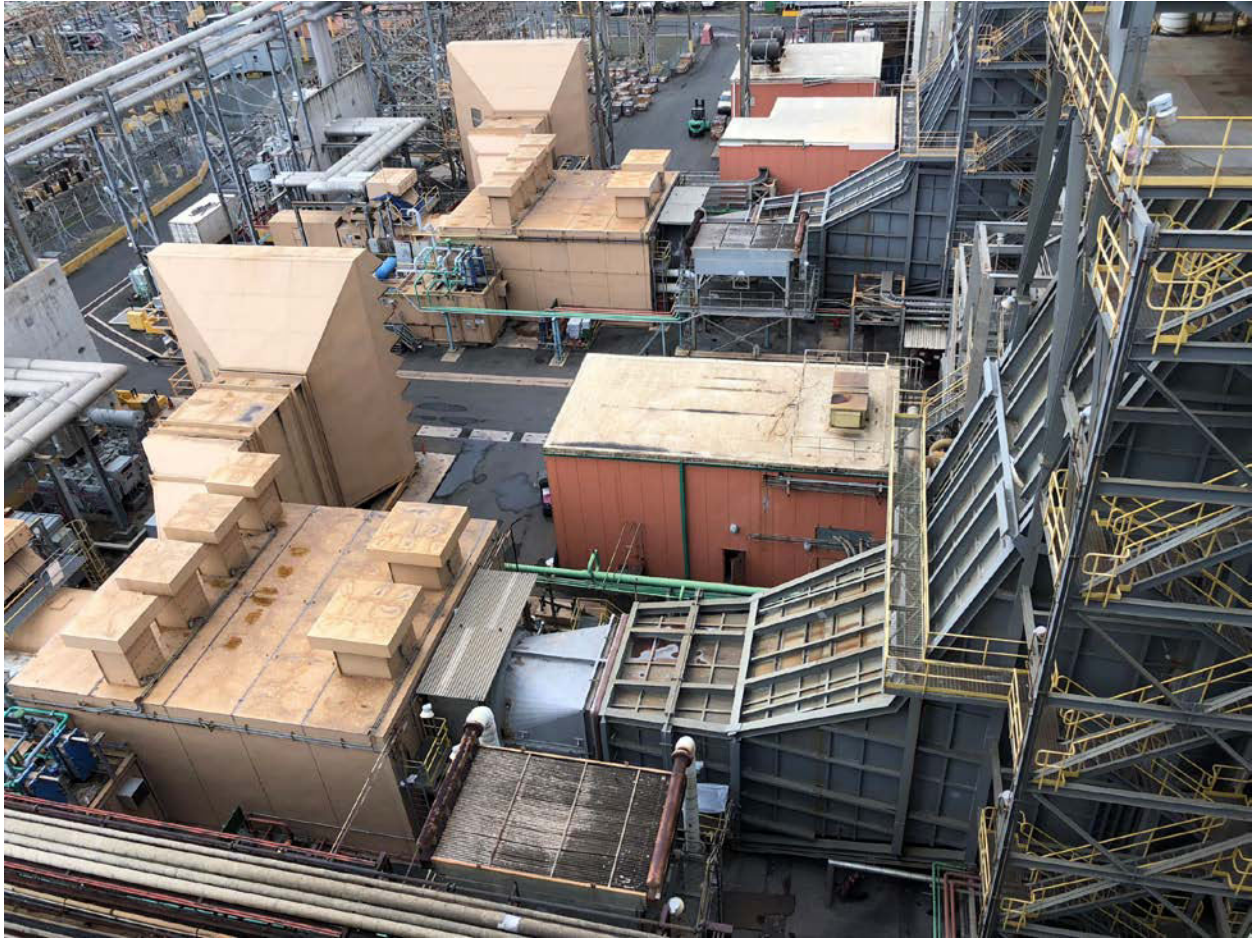
Figure 2-3 - San Juan Units 5 & 6 Combustion Turbines
