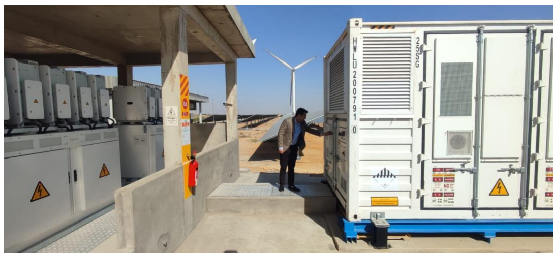
Figure 18: BESS with Power Conversion System (PCS)
