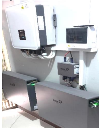
Figure 13: Bilal's Residential BESS System
