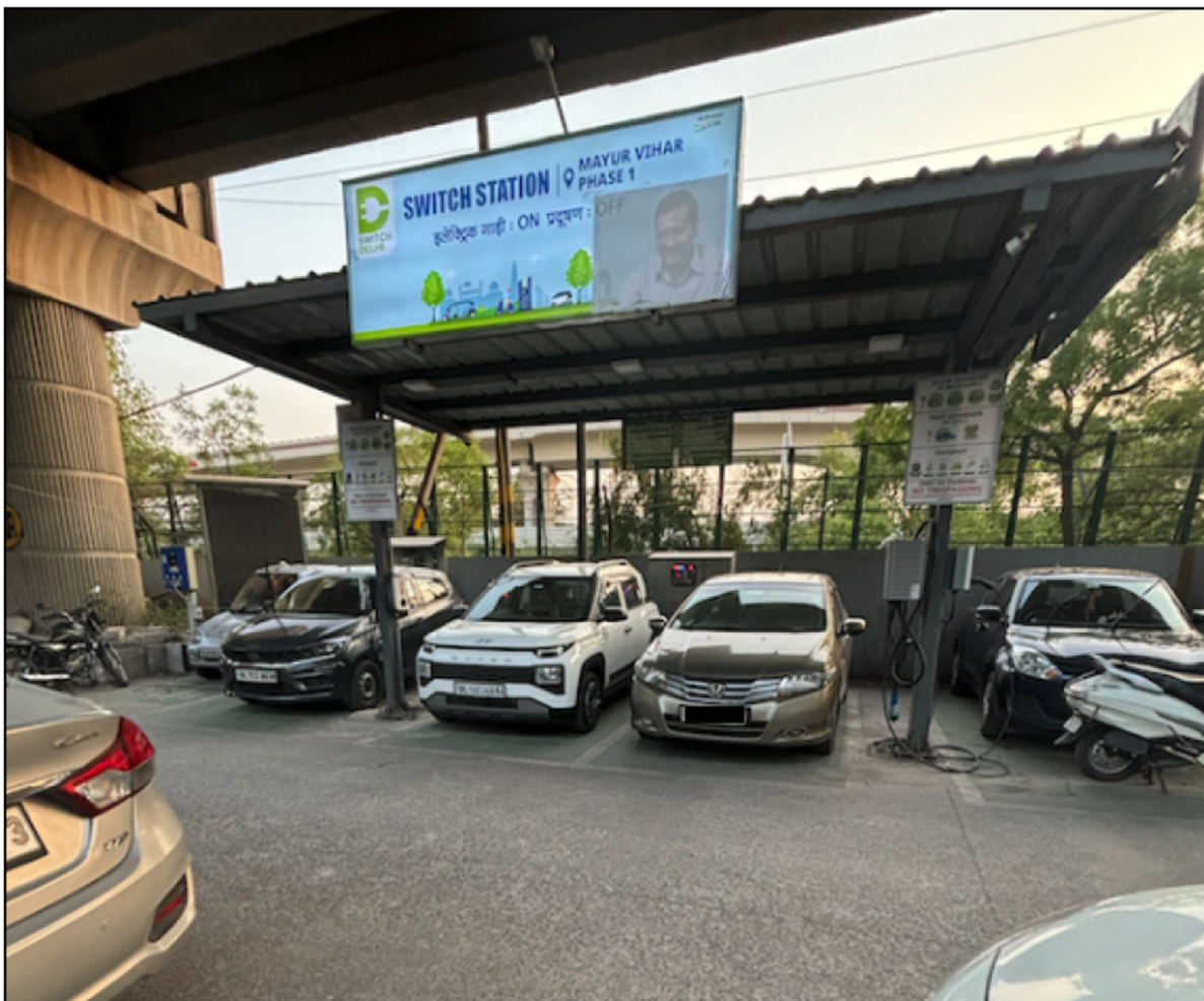
Photo 4: Functional but inaccessible chargers at Mayur Vihar Phase 1 Metro Station
