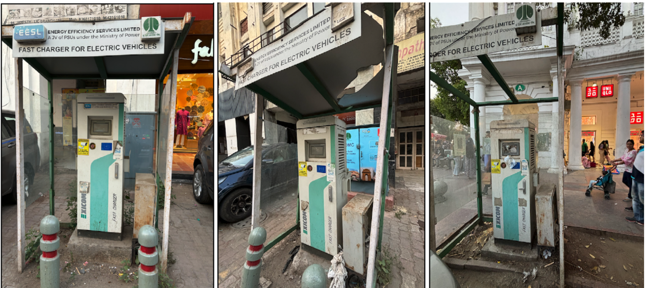
Photo 2: Non-functional EV chargers in Connaught Place, Delhi
