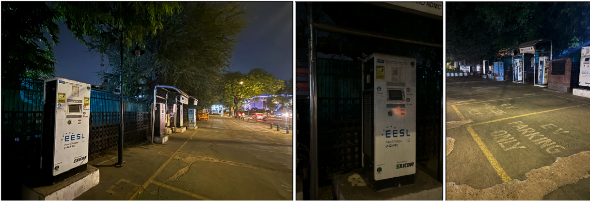
Photo 3: Non-functional EV chargers at Patel Chowk, Delhi
