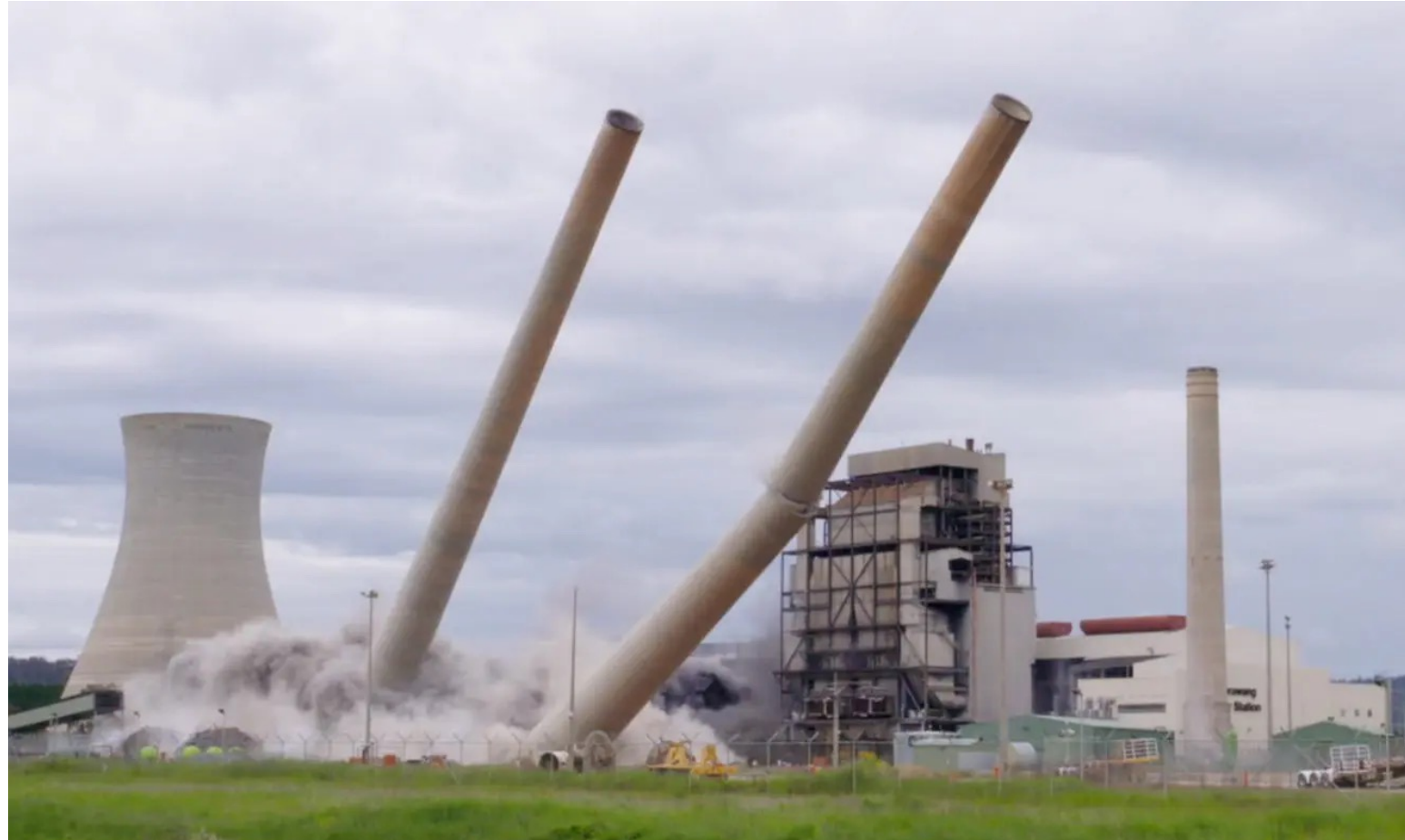
Wellerawang coal fired power station (credit: Greenspot/Liberty Industrial)
